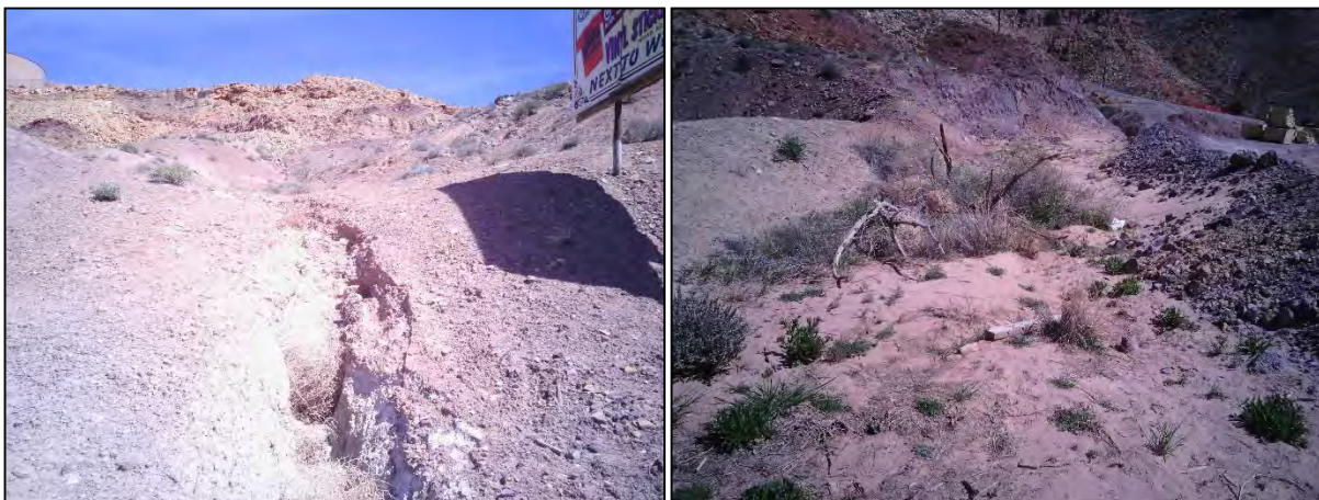
Steep Unconsolidated Soil Erosion
